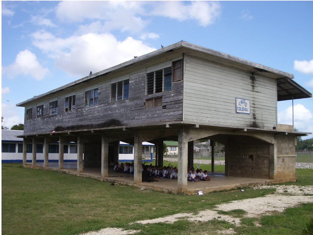
Plate 7: Two-storey classroom building; note heavy RC frame to ground floor and water-damaged walls and rusting louvre windows to first floor.
