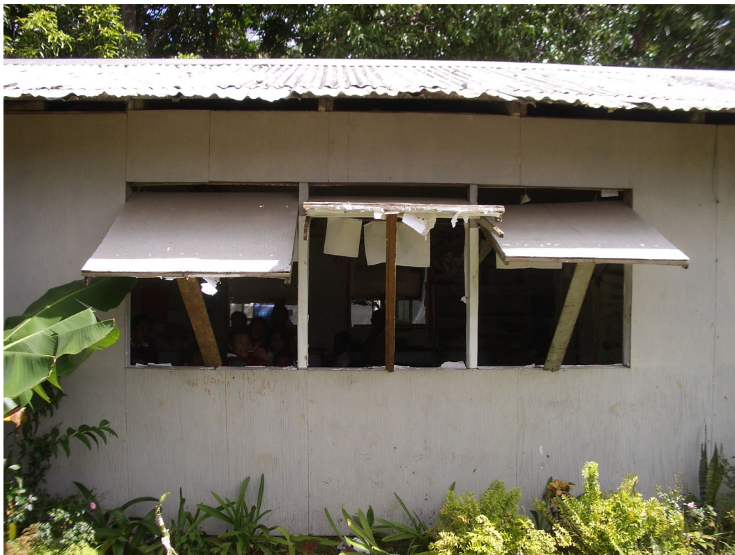
Plate 2: Classroom Building 2 showing very poor roof construction and top-hung shutters
