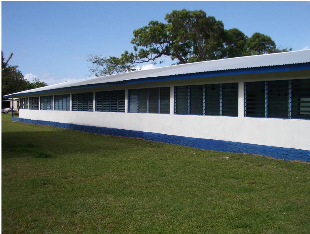
Plate 6: Badly constructed and poorly renovated single-storey classroom building.
