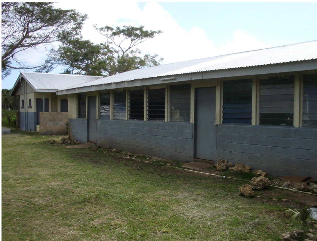
Plate 4: Rear elevation of Classroom Building 2; note timber frames supporting roof and sitting on top of block wall; these frames are not secured to the wall.
