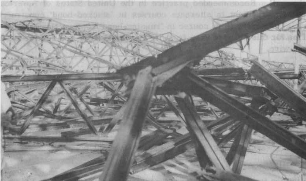
Plate 7. Steel frame failure from strong wind.
