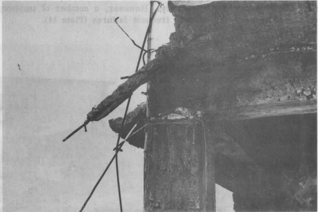
Plate 12. Exposed reinforcement in the underside of the concrete roof of this school is a factor contributing to failure of the slab.
