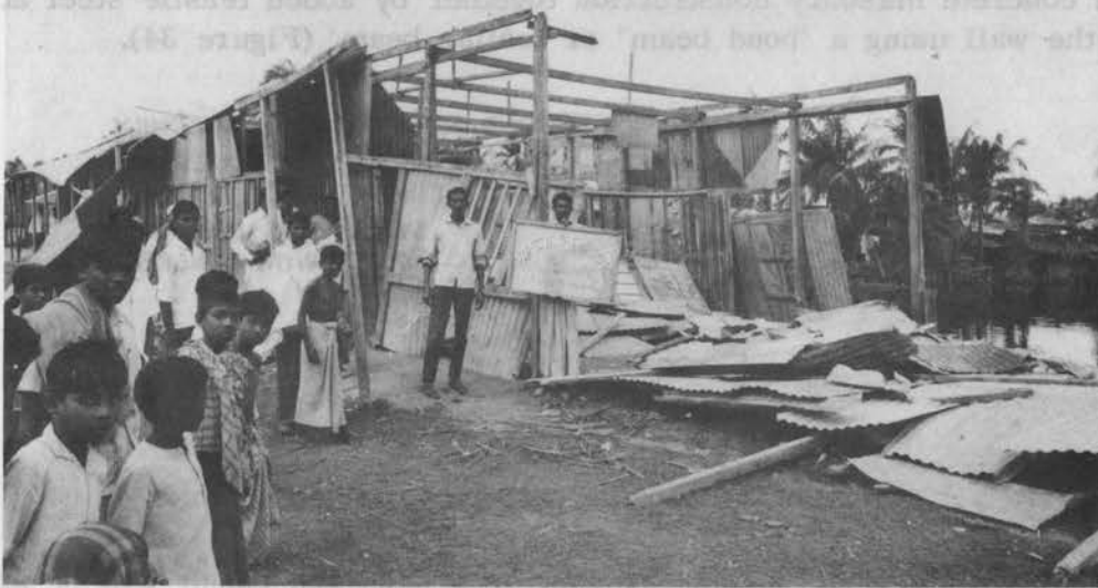
Plate 6. Timber frame failure from strong wind.
