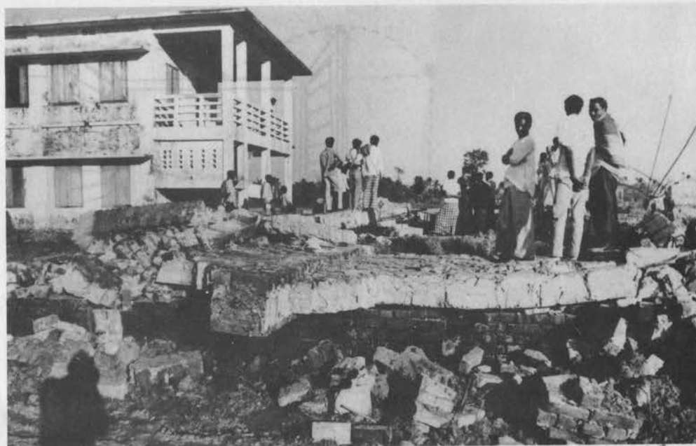
Plate 8. Shutters and frames in the two-storey building have successfully withstood the cyclone that has just destroyed the school building in the foreground.
