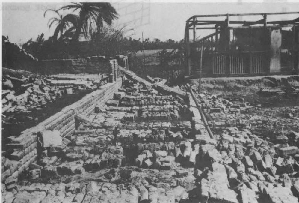
Plate 5. Masonry wall of a school building that failed in the Bangladesh 1970 cyclone. The angle of the trees suggests the wall collapsed due to negative pressures.
