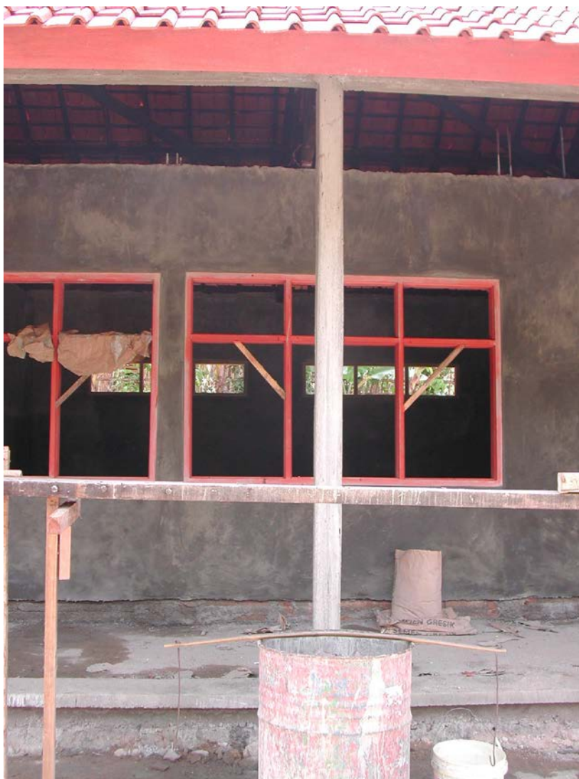
Plate 1: SDN Gendaran 01 showing inadequate column sizes, lack of intermediate columns to classroom wall and trusses over the centre of windows
