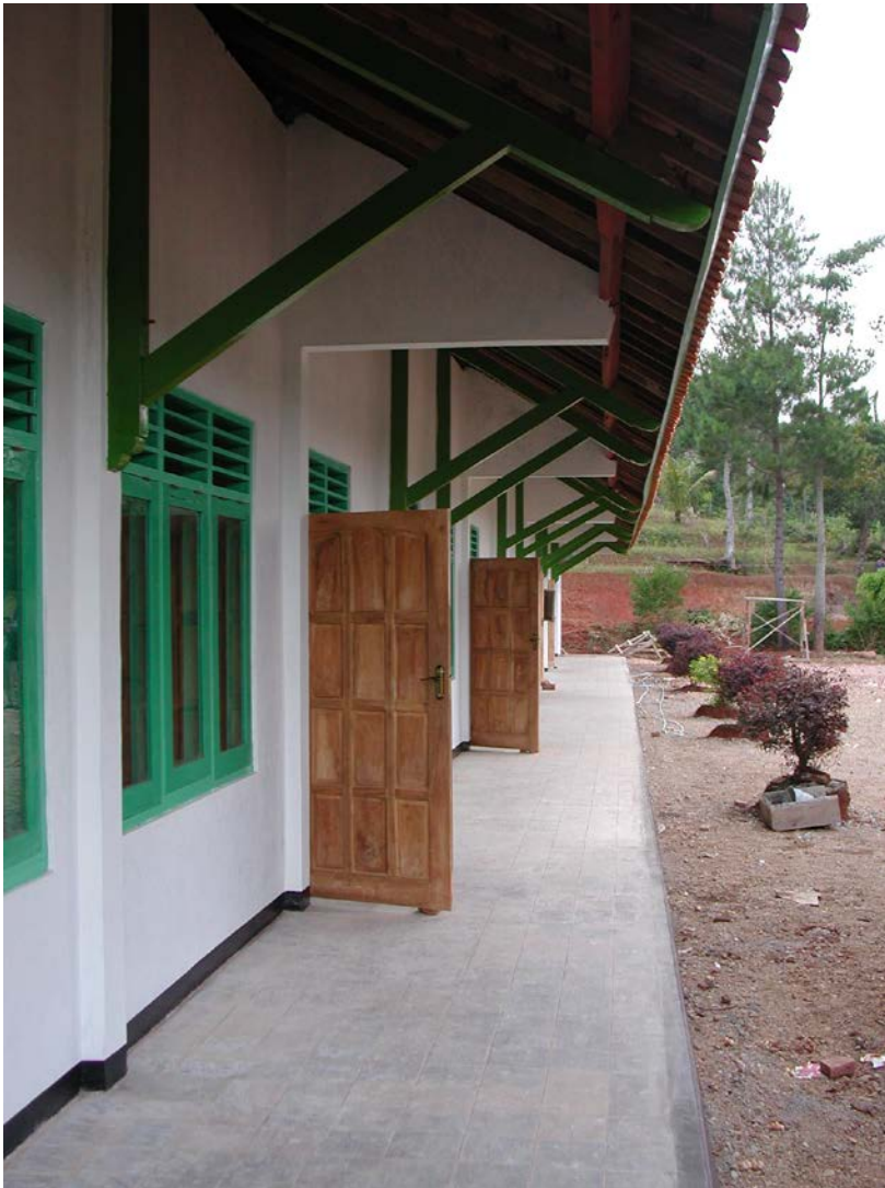
Plate 7: SDN Tahinan 5 showing concrete cantilevered beams the structure of which should be checked
