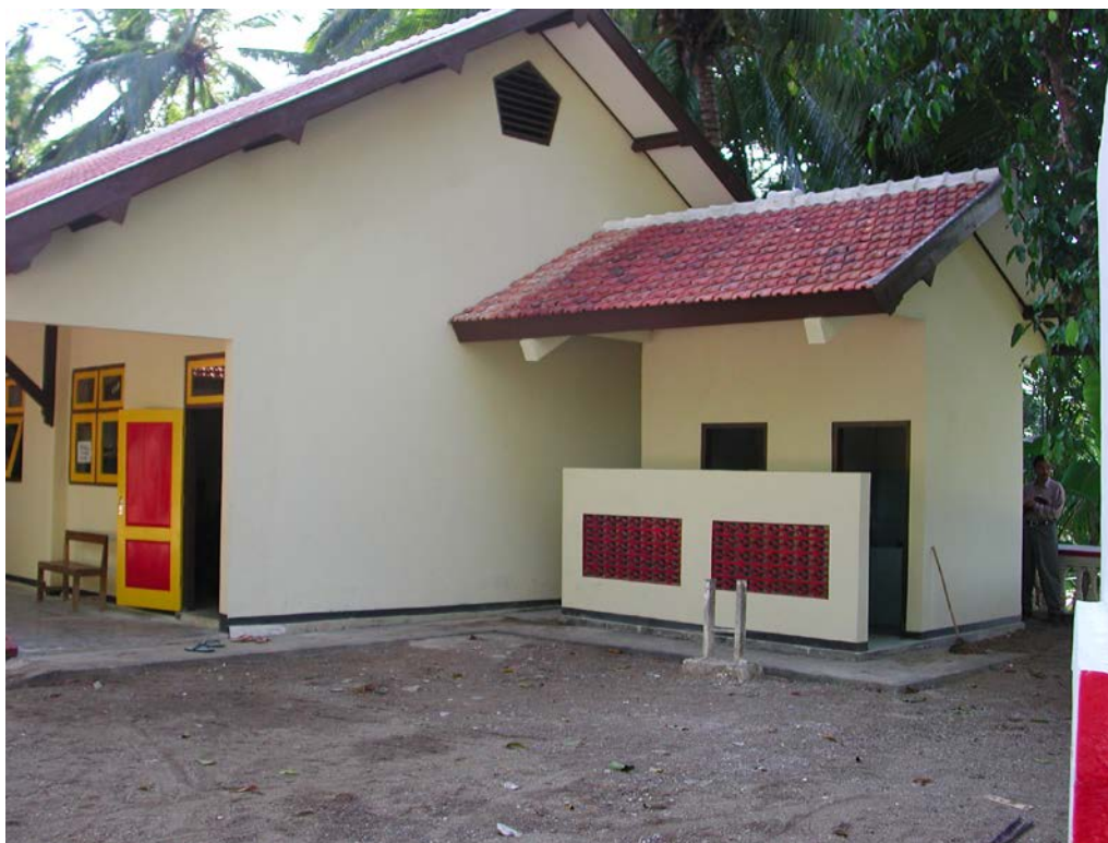
Plate 17: MI Guppi showing new toilets and large RC cantilever beams that should be checked
