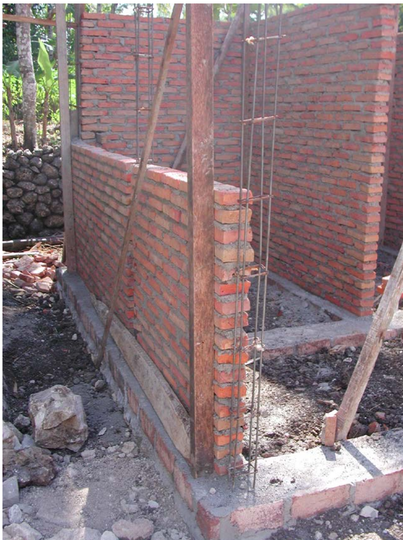
Plate 2: SDN Gendaran 01 showing inadequate column sizes to toilets
