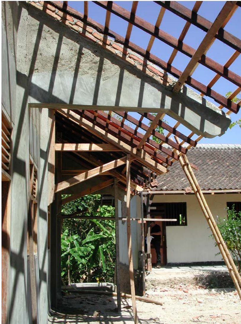
Plate 3: SDN Sendang 3 showing large concrete cantilevers, the structure of which should be checked
