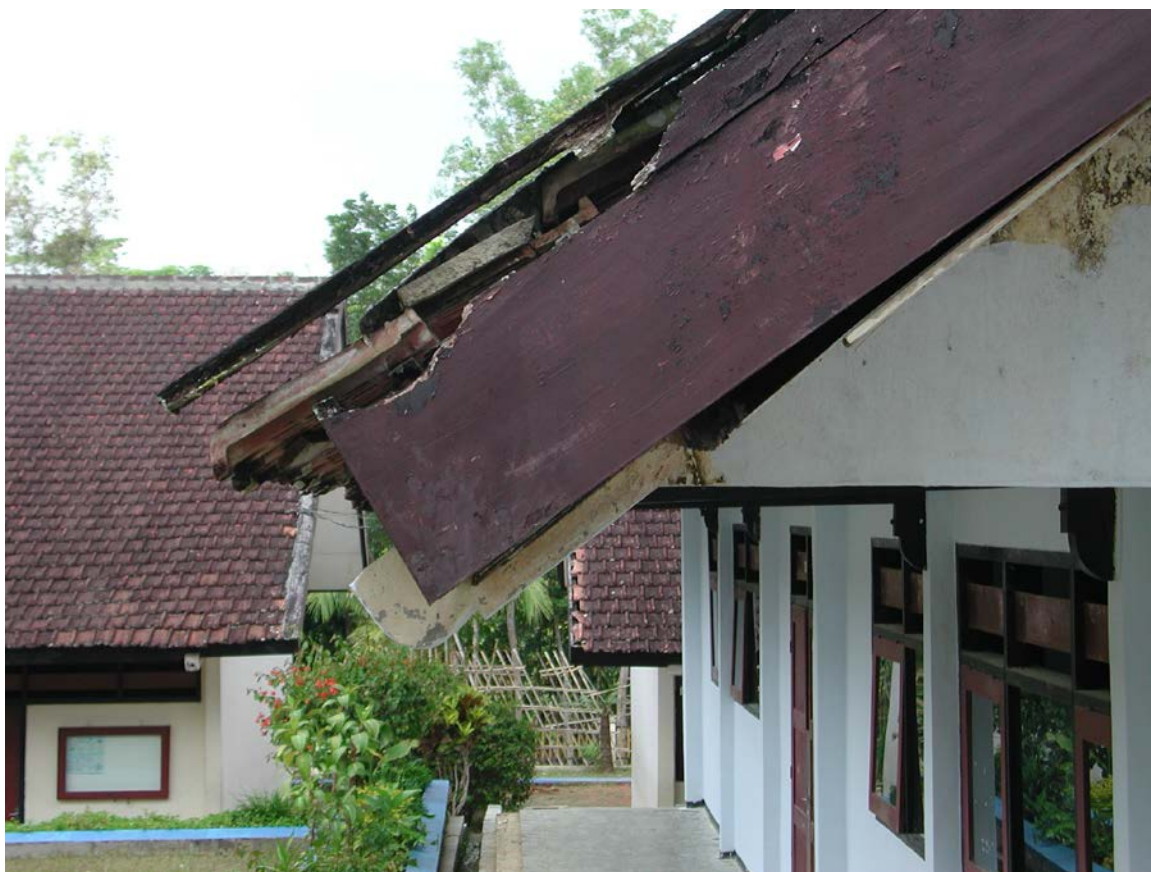
Plate 13: SLTPN 2 Tulakan showing typical roof that requires urgent repair
