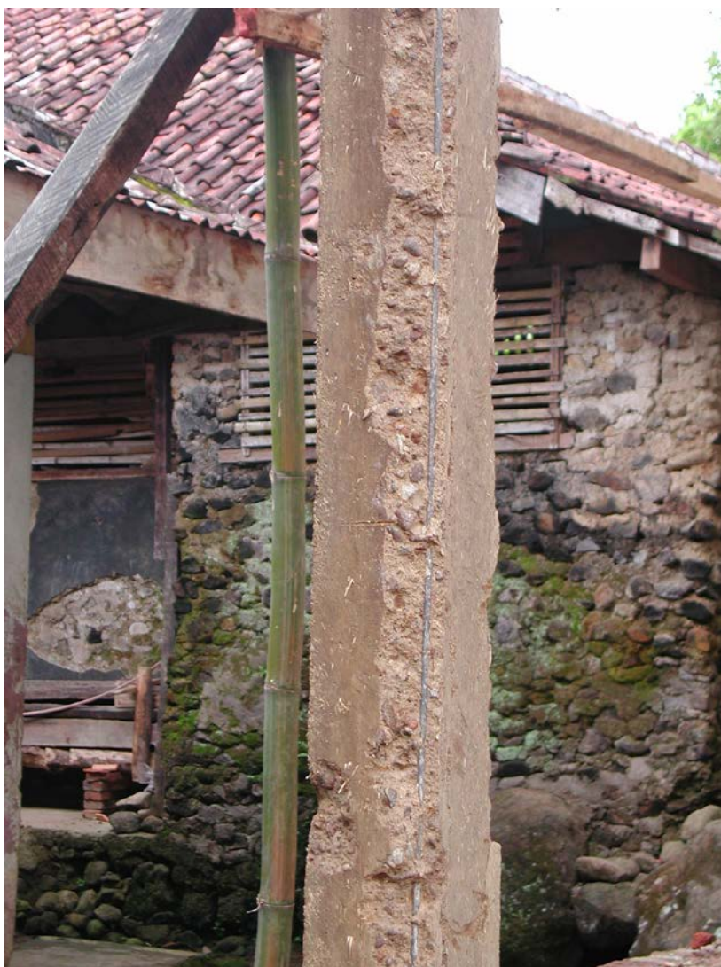
Plate 8: SDN Banjar Negara 1 showing very poor concrete
