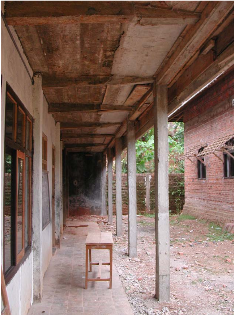
Plate 8: MTs Al-Fatah showing inadequate ground floor structure
