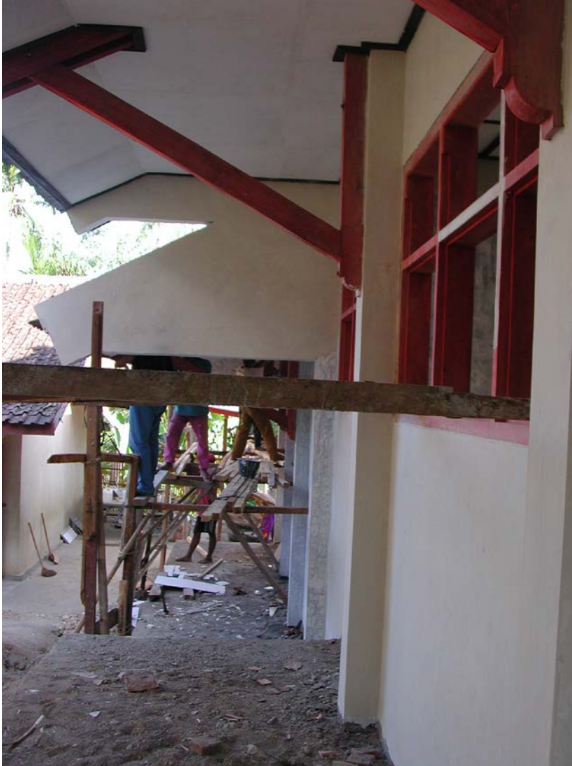
Plate 5: SDN Gungangan 02 showing large concrete cantilevers, the structure of which should be checked
