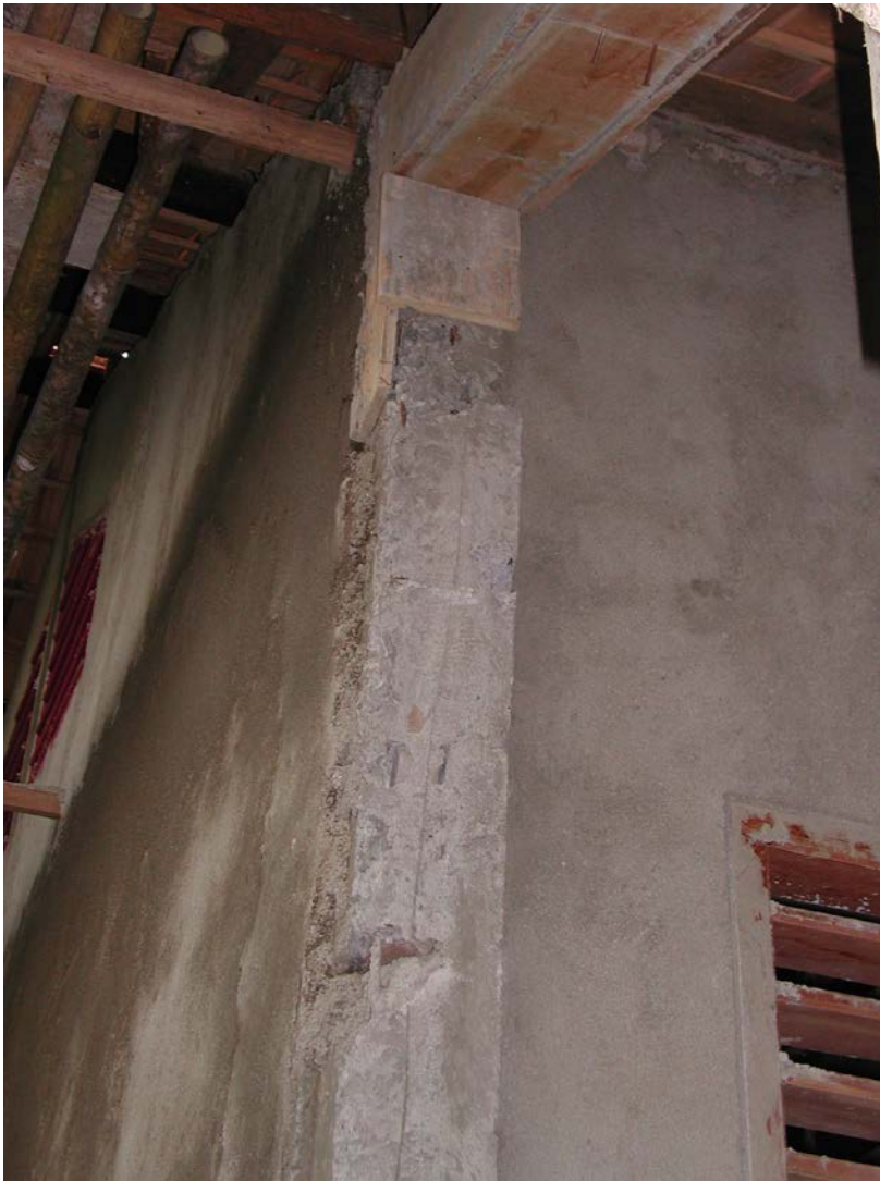
Plate 4: MIs Al-Ishlah Laksana showing poor quality concrete
