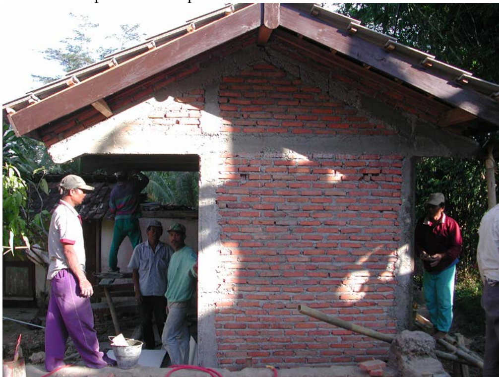
Plate 4: SDN Gungganggan 02 showing cantilevered roof to toilets with only 6mm reinforcement
