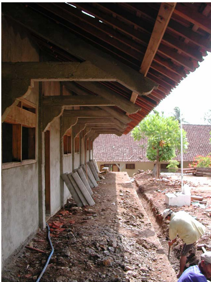
Plate 12: SDN Ketro 2 showing RC cantilevers to veranda that should be checked
