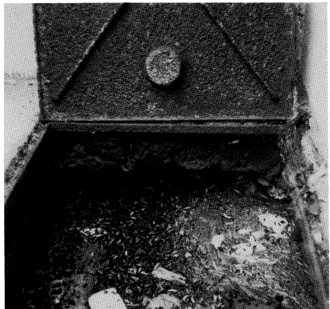
Figure 6 Cockroaches and fly larvae in poorly sealed aqua privy tank
