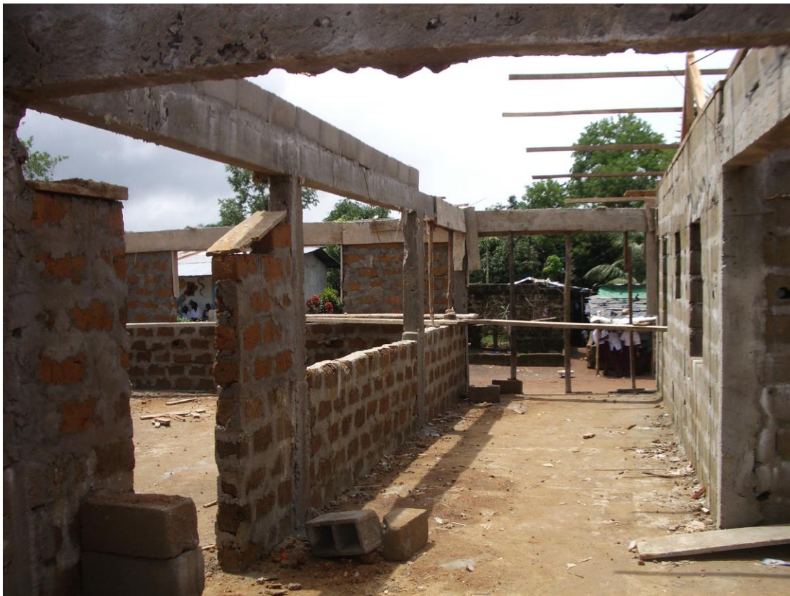
Plate 1: Sarah Barclay Elementary School showing one of the new buildings: note the mud bricks and poor quality concrete
