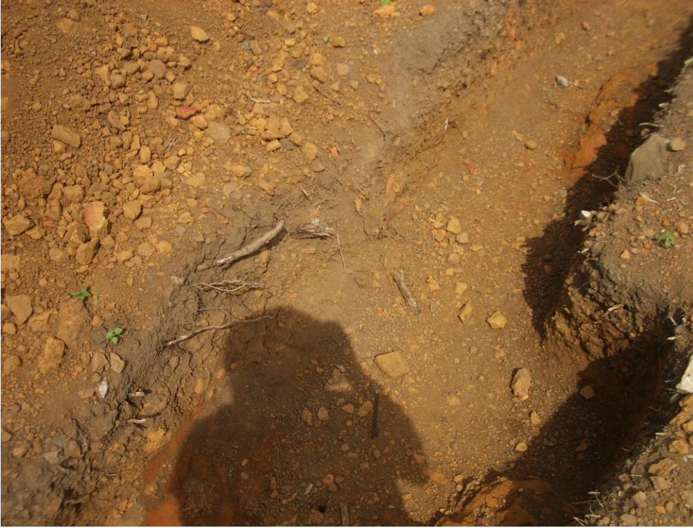
Plate 2: Rehab Community Primary School showing root in foundation trench
