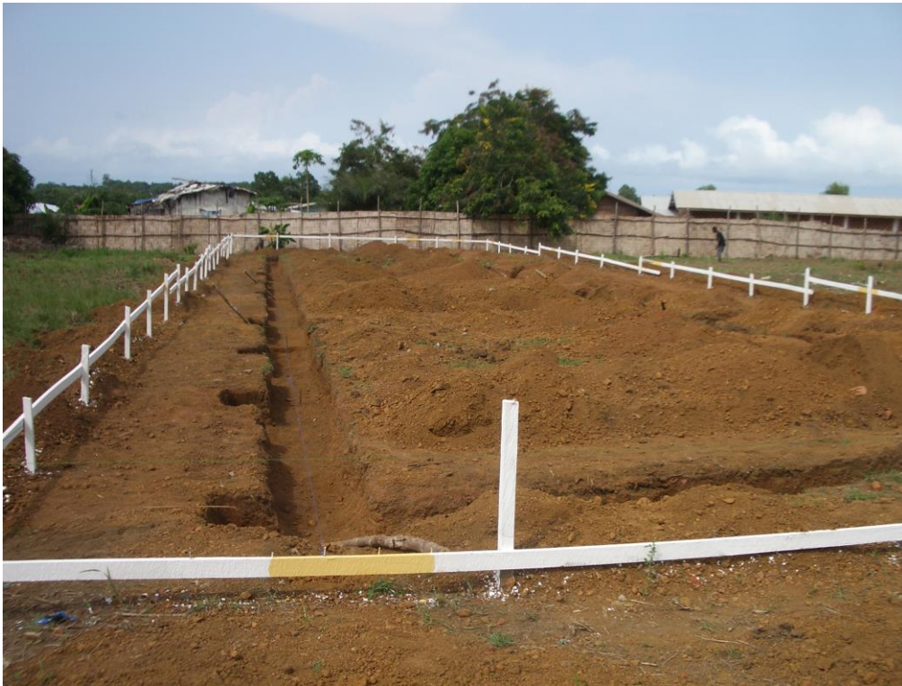
Plate 1: Rehab Community Primary School showing very shallow foundations
