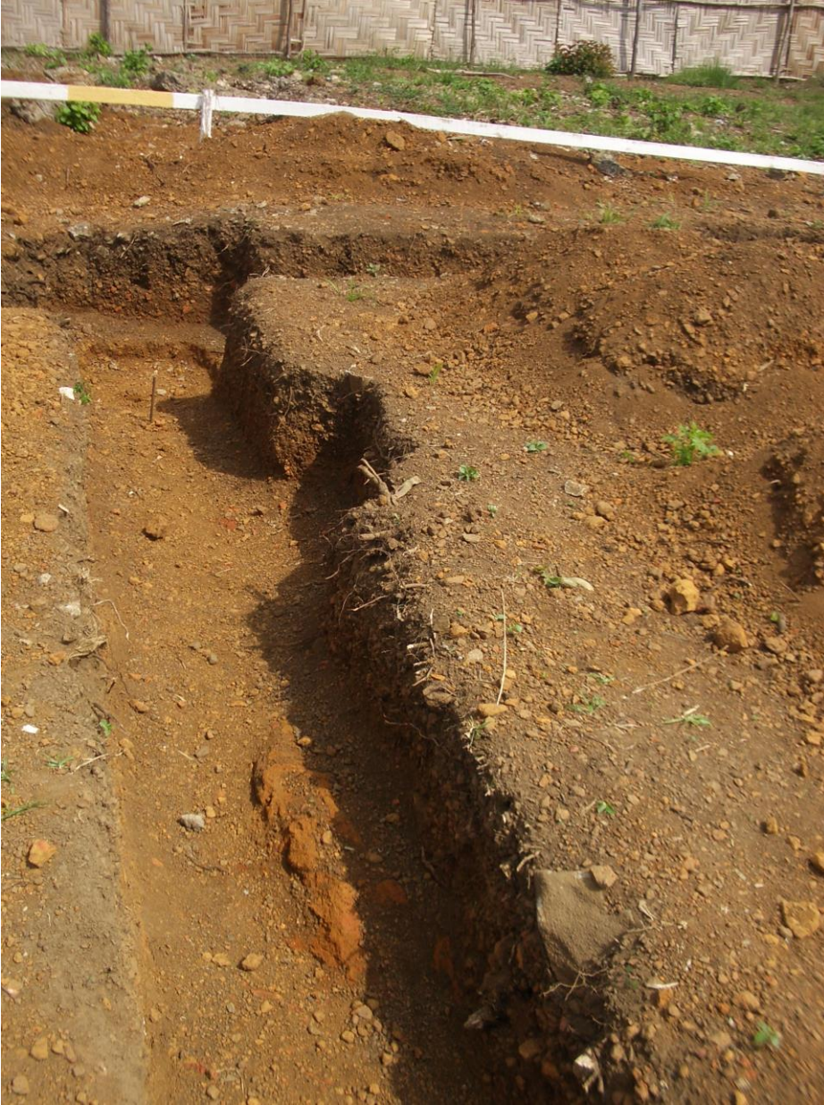
Plate 3: Rehab Community Primary School showing vegetable matter and topsoil that has not been stripped off the area of the buildings and rock in the foundation trenches.
