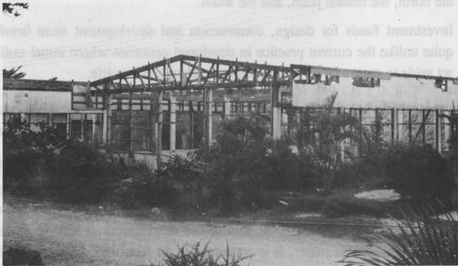
Buildings damaged by Typhoon Gay on 3 November 1989
