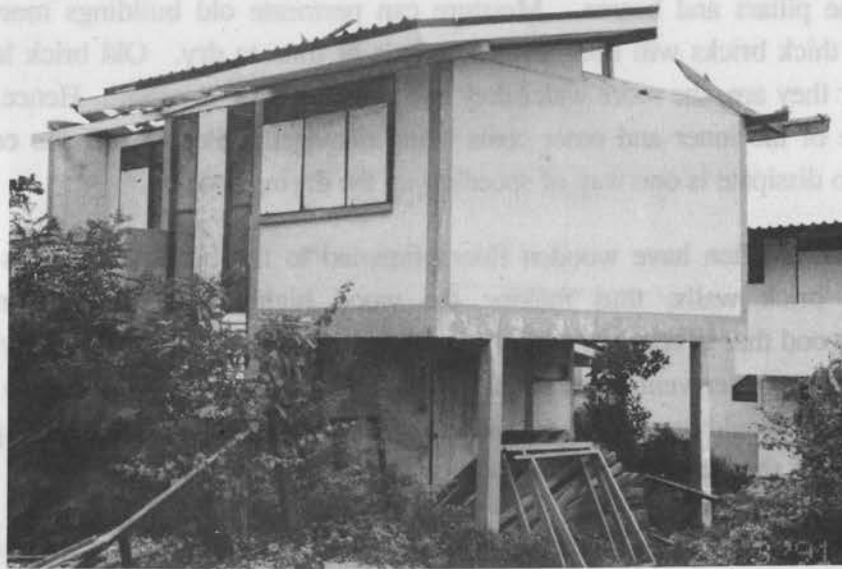
Buildings damaged by flood and wind
