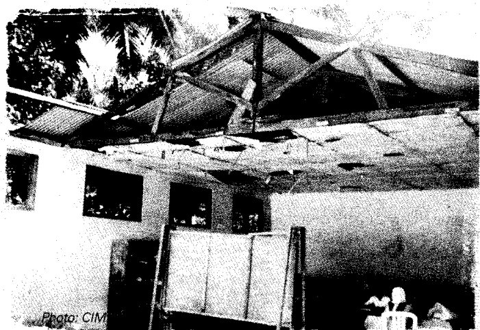
Students in SDN Kadu Agung Barat 3 take their lessons in this severely damaged classroom. The ceiling is in a state of total disrepair not only making this classroom impossible to use during rains, but also putting students at risk if any more of the structure should collapse.
