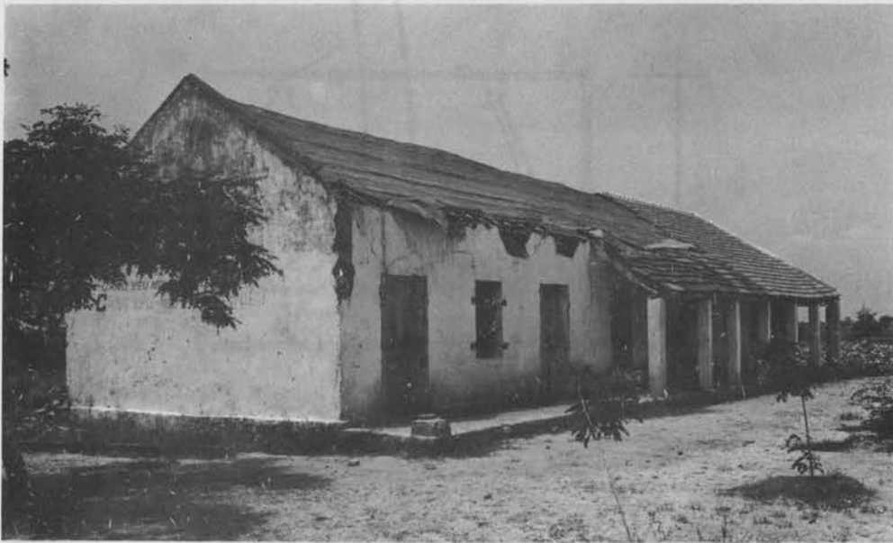
Fig. III.9 Doors and windows with hinges attached to walls, unable to resist strong wind.
