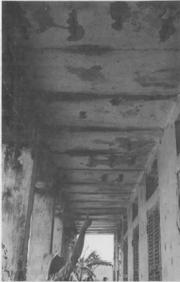
Thin RCC slab. There is no cover to protect reinforcement rods. Thus rust attack has led to expansion of the rods and cracking of the concrete. See also below.
