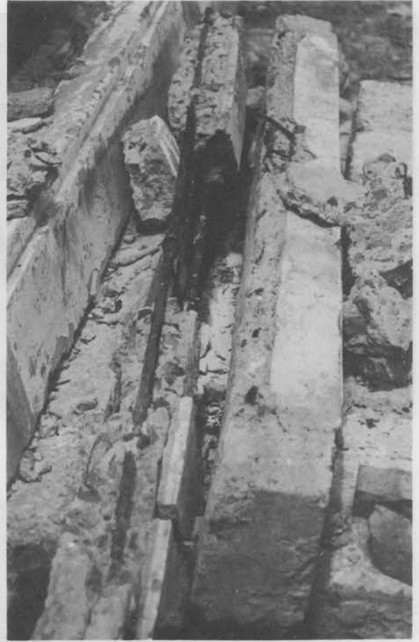
Precast columns or slabs removed from building because they were attacked by concrete cancer. Materials must be free of impurities such as salt which causes steel to rust.
