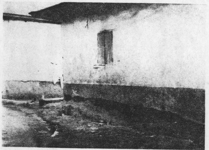
Fig. 2. Erosion at the base
