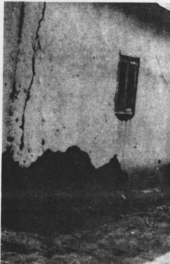
FIG 2B. Erosion of a foundation of an earth building due to short eaves overhang and lack of concrete platform.
