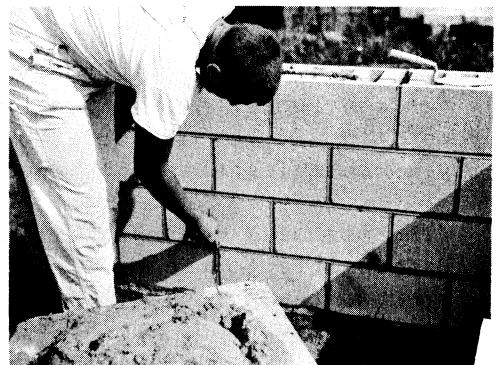
Tool the horizontal joints first, then strike the vertical joints with a small S-shaped jointer.
