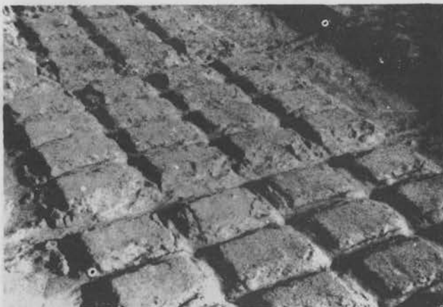
Figure 47. Inadequate protection of blocks during curing schedule may result in a loss such as occurred here after a rainstorm.
