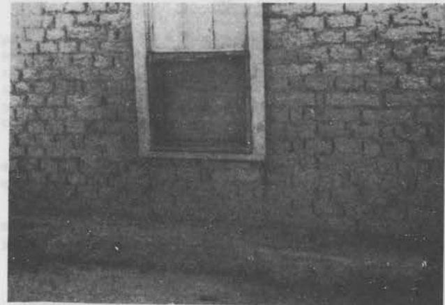
Figure 66. An overhanging window sill channelizes the rain into two rivulets, easily eroding the unprotected, nonstabilized wall surface.
